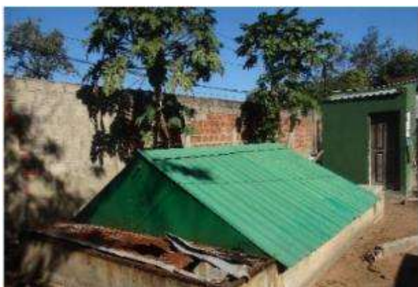
Public toilet and biogas unit as a septic tank. Manhica.
