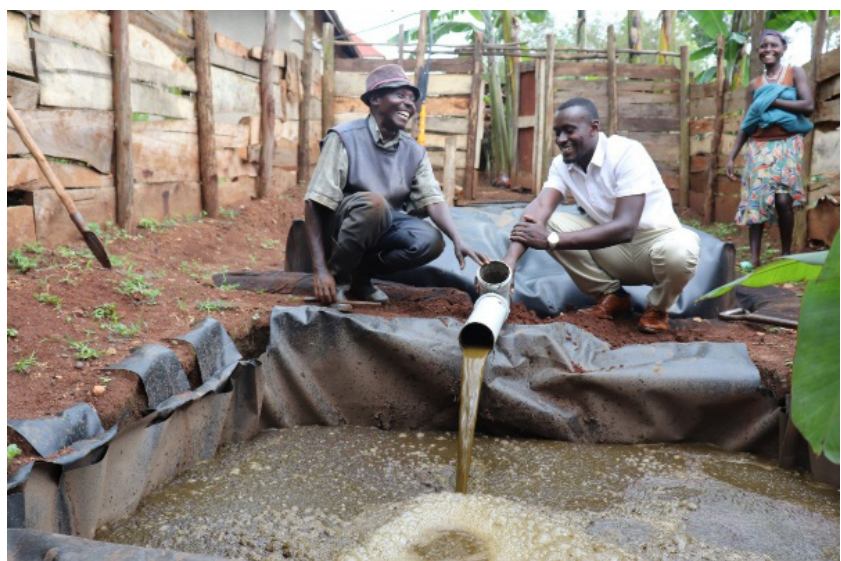
Herbert Murungi (centre), RESI Manager, helps to unclog the bio-slurry pipe in Katooke village, Kyenjojo District.
