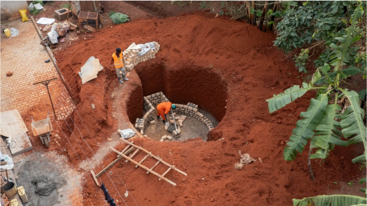
A biogas digester in Kawempe, Kampala being constructed as per the new Biogas Digester Construction Guidelines ©GIZ/Uribi Media
